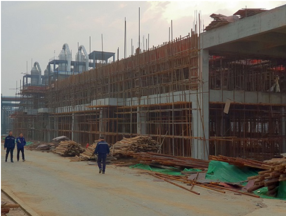
Ongoing construction for hydroxide circuit in the foreground with existing leach circuit in the background at Jiangte's Yinli New Energy facility
